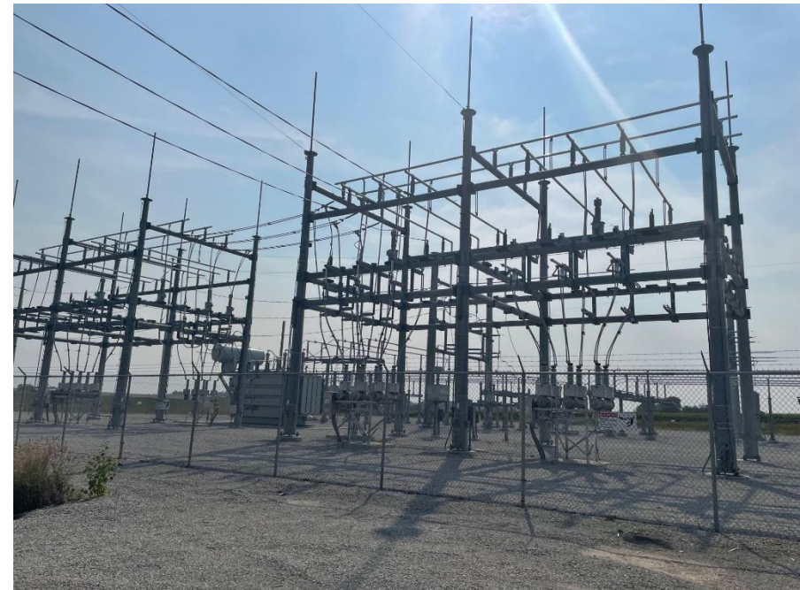
CIPCO's Swan Lake substation near North Liberty
