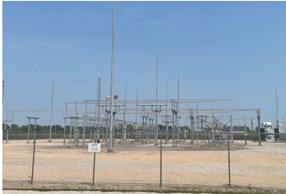
ITC Midwest's Fairfax substation near Fairfax
